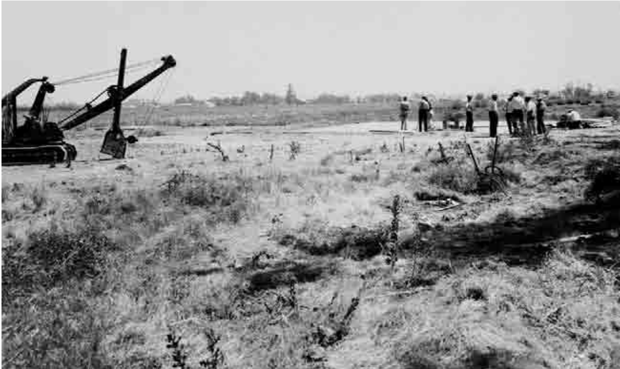
A few days after the official groundbreaking ceremonies on August 15, 1930, the hard work of building a hospital begins with just a few engineers and architects standing in an open field. The nearby crane awaits. (Photo courtesy of the San Bernardino County Museum, from the Steele collection.)
