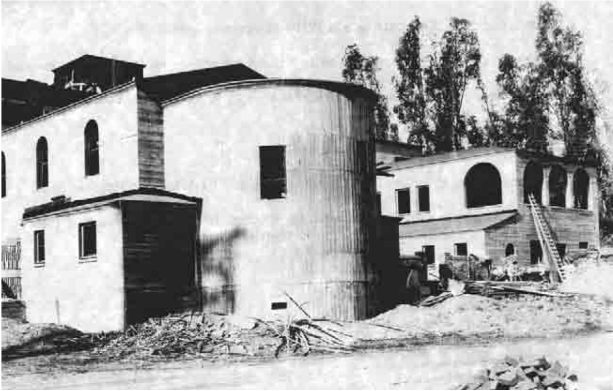
The new St. Bernardine Hospital Convent under construction in the winter of 1930. ( St. Bernardine Medical Center archival photo. )
