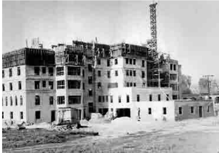
Construction of the main hospital, viewed above from the back, continued in 1931 until its dedication in October of that same year. (Photo courtesy of the San Bernardino County Museum, from the Steele collection.)
